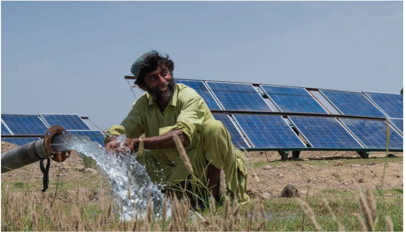
A solar irrigation system developed by Jalwala Village Organisation at Killi Jalwala, UC Phelawagh, Tehsil Phelawagh, Dera Bugti
